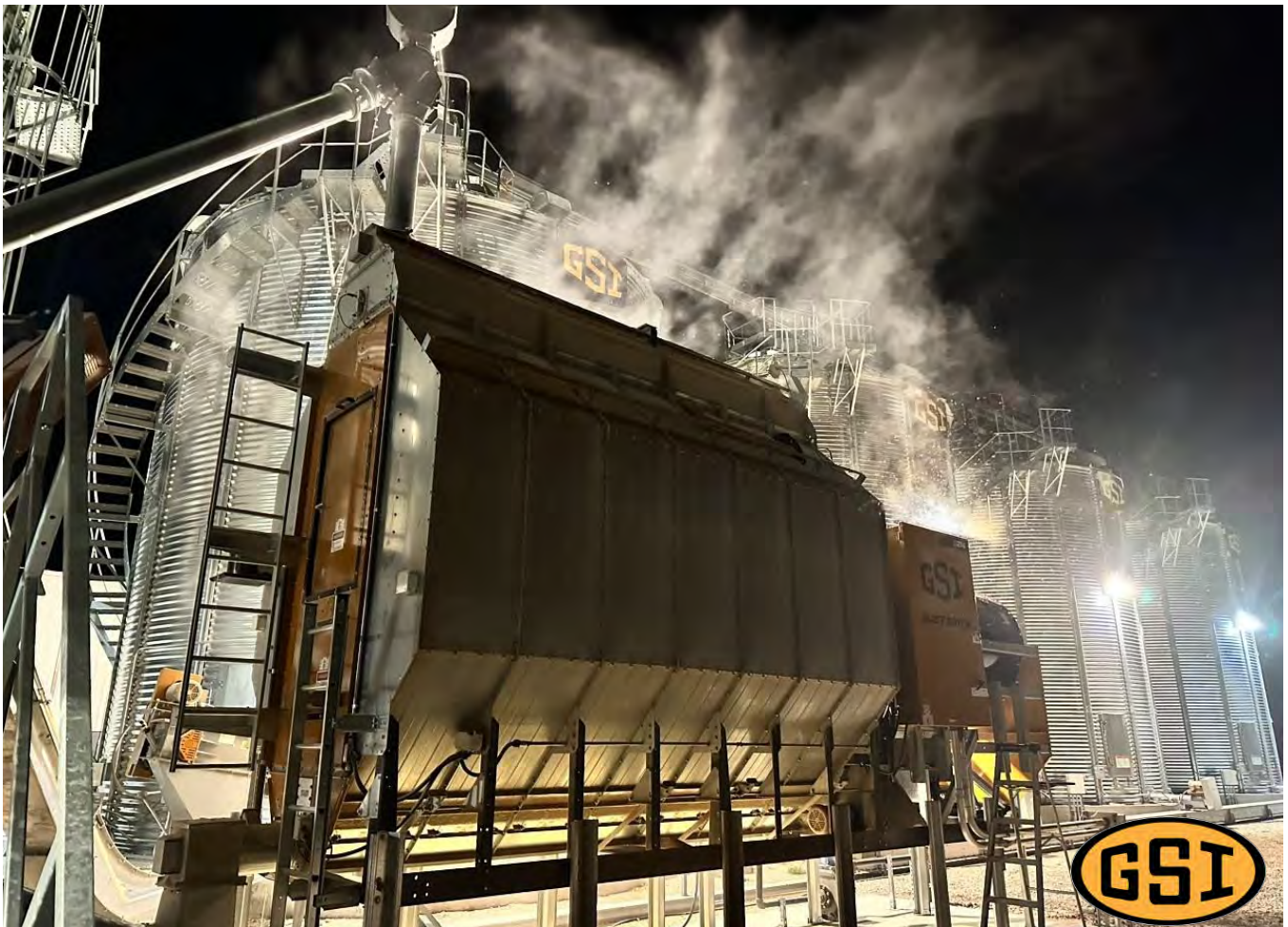
Figure 1. GSI Grain Storage Facility with Q214 Quiet Dryer
